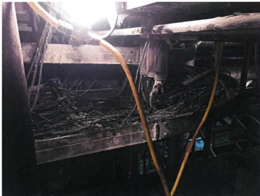
Figure 1: Fire damage to cables and cable tray
